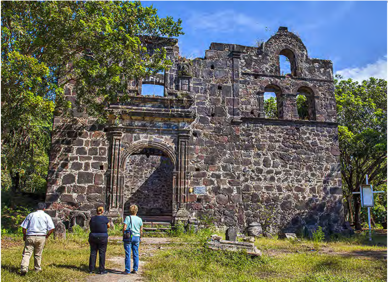
The bones of San Blas' oldest church, Our Lady of the Rosary, built on San Basilio hill in 1769 and a romantic destination for weddings, need a roof, door and windows to come back to life. Memorialized by Henry Wadsworth Longfellow, in his poem "the bells of San Blas," it's San Blas' most popular tourist attraction. Photo by © Haggerty/ColorWorld.
